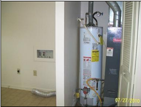
Hot water heater & Furnace in closet INSIDE the home; no crawling under the house to change filters!
