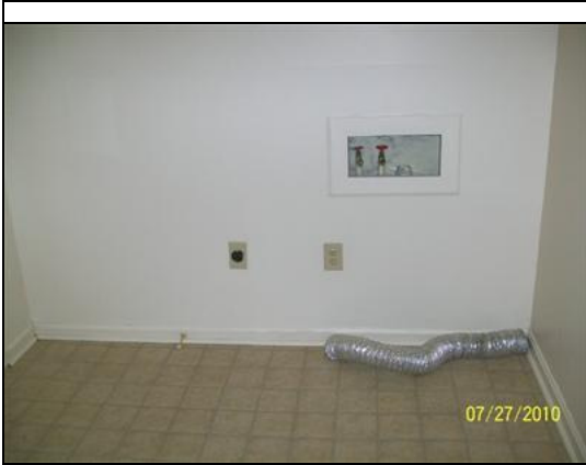
Washer & Dryer area, out of the way to one side of Kitchen!
